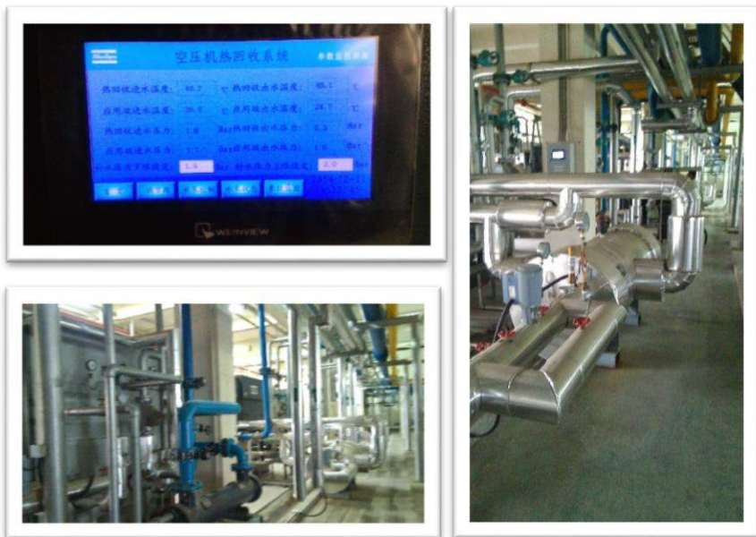
Energy saving project of air compressor system
