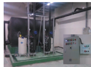
Recycled water dosing treatment
